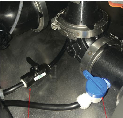
Figure 70. Vannes de vidange
